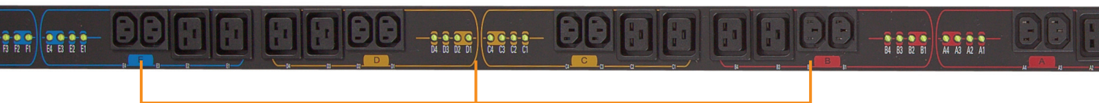
Outlet number identifications are color coded to match the outlet section to the appropriate circuit breaker.
