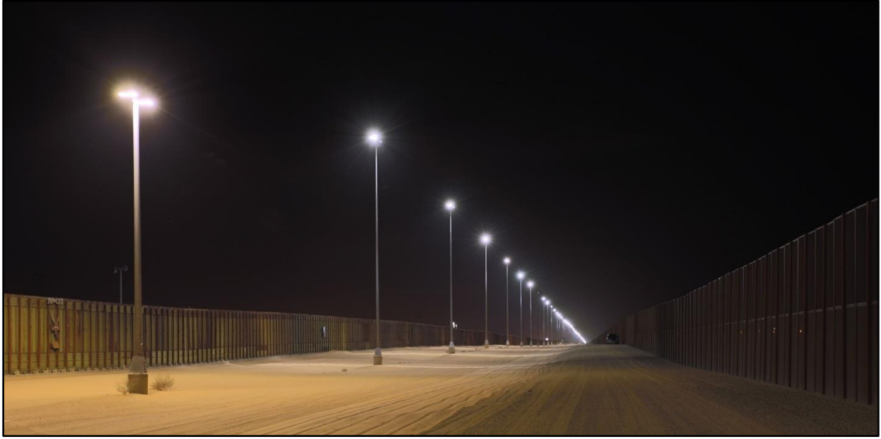
Figure 4. Trial Demonstration Site on the U.S.-Mexico Border: Nighttime. The 24 ft difference in height is visible in this image. The primary fence is on the left and on the right is the secondary fence—less noticeable in this image due to the relatively low light level on the fence.
