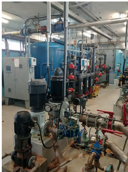
Nordikeau is using Fetch Data Collector to view real time data from critical assets at a water treatment plant in Canada
