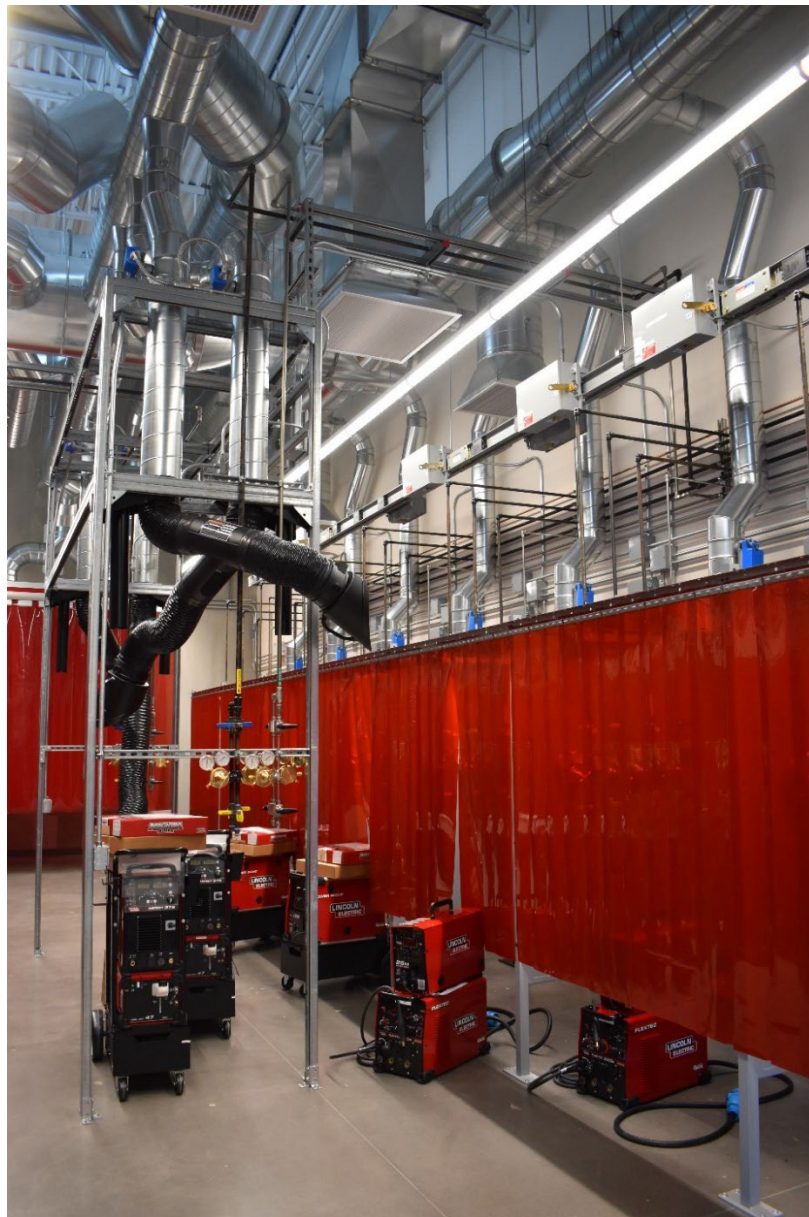
Welding booths, Oregon Manufacturing Innovation Training Center at PCC Columbia County Center.
