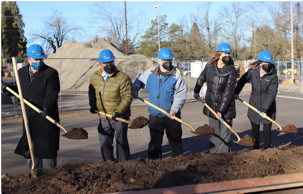
Portland Community College leaders, college partners, and local leaders officially broke ground on PCC's 50,000-square-foot Opportunity Center , which will feature extensive sustainability aspects as it aims for LEED Gold certification.
