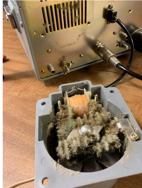
Before Cleaning FT-101ZD Rear Panel and Fan Showing Lint in Fan Assembly
