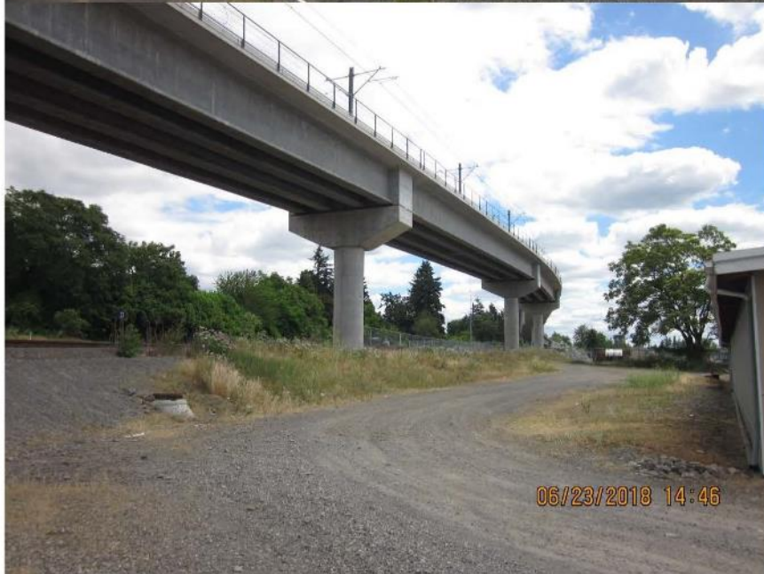
Milwaukie Light Rail Orange Line Segments near SE Ochoco Street Industrial Area.
