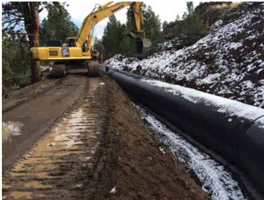
Figure 6-2. An Example of Construction on a Tumalo Irrigation District Lateral using an Existing Maintenance Road.
