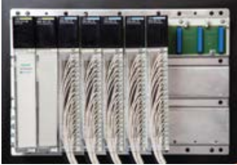
Existing Control System
