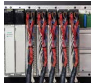
Completed & migrated DCS system
