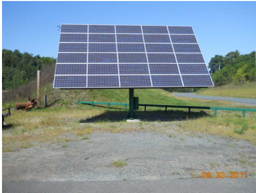
Figure 3-15. Tracking Solar PV Array, Renewable Energy Program Area
