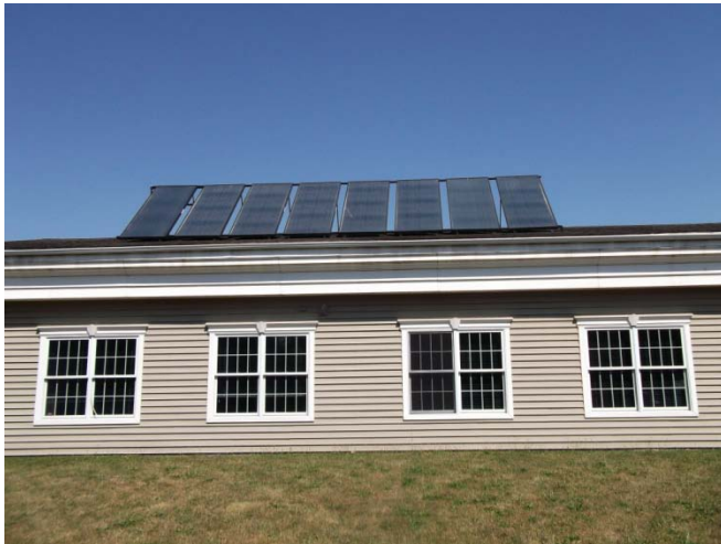
Figure 3-12. Roof-Mounted Solar Collectors at SHW System, Renewable Energy Program Area
