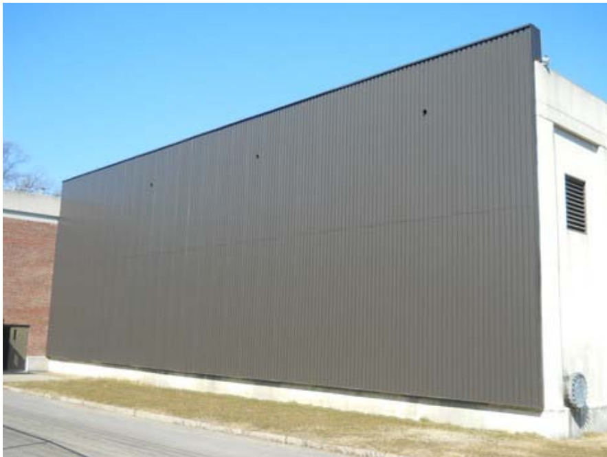
Figure 3-6. Monitored Solar Wall Project, Renewable Energy Program Area
