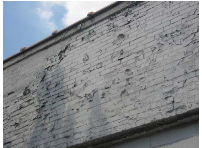
16. View of peeling exterior paint on the subject property building.
