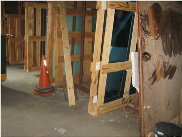
13. View of the area of the USTs along the southern interior wall of the site building.
