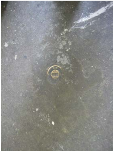
9. View of the fill port associated with one of the on-site USTs.
