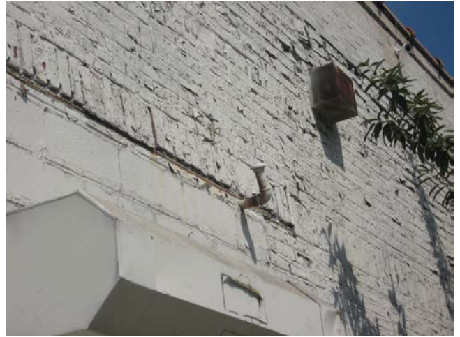
2. View of the vent pipe observed on the east exterior wall of the site building.
