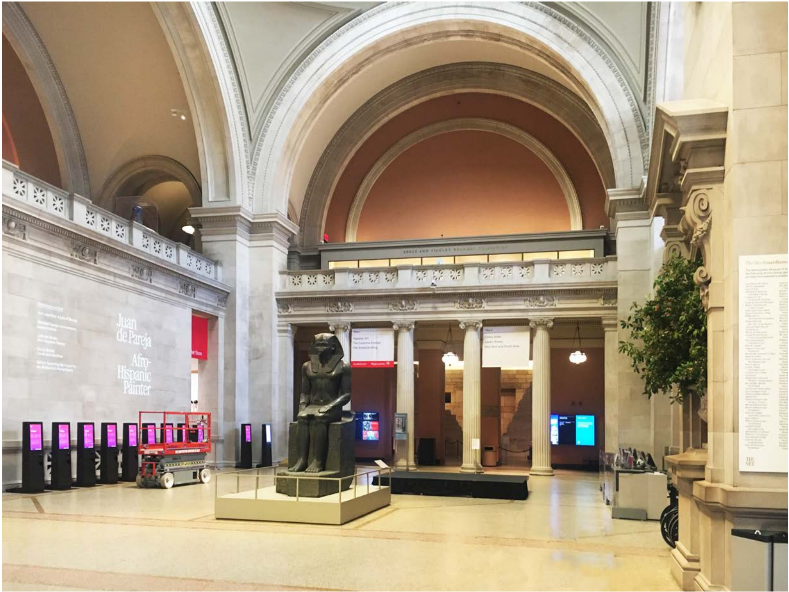
PHOTO OF TEMPORARY DISPLAY SCREEN INSTALLATION, LOOKING NORTH
