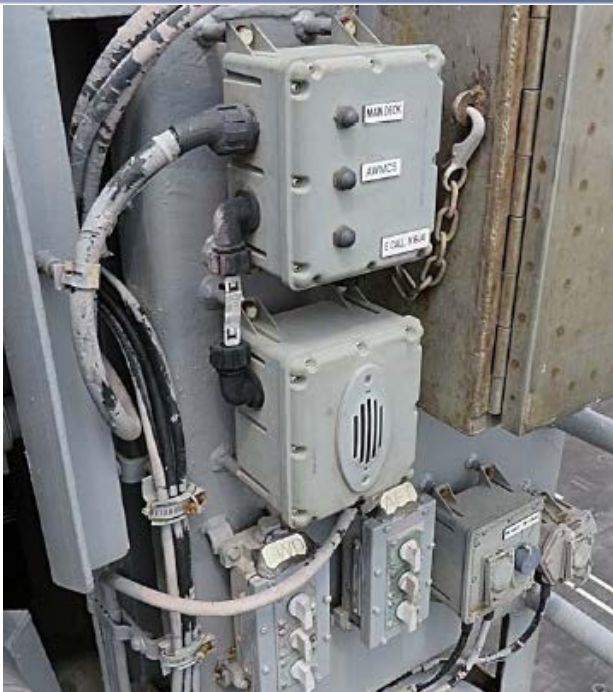
CVN Aircraft Elevator Station
