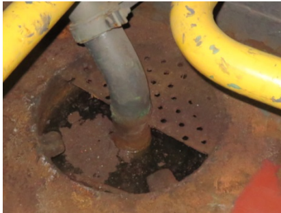
LHD well deck grating
