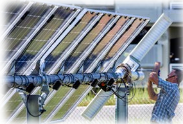
(Photo by Werner Slocum / NREL)
