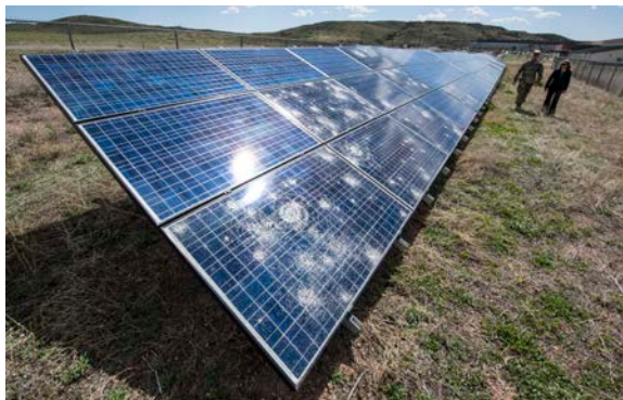
PV modules damaged by hail (Photo by Dennis Schroeder / NREL)
