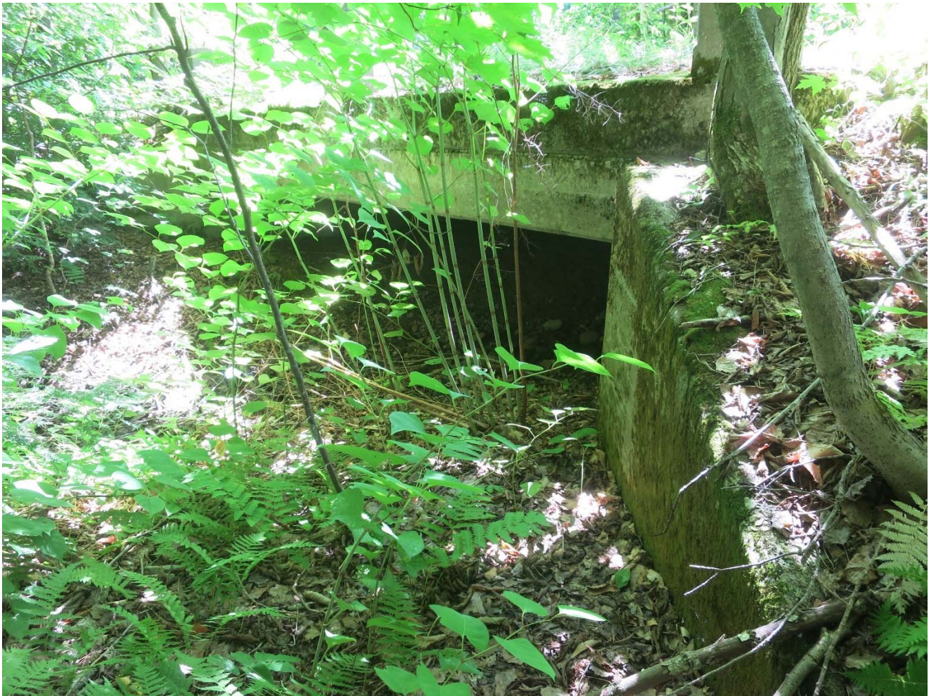
11. View of the small approach bridge, showing its north façade and one of two wing walls, looking south, August 2022.
