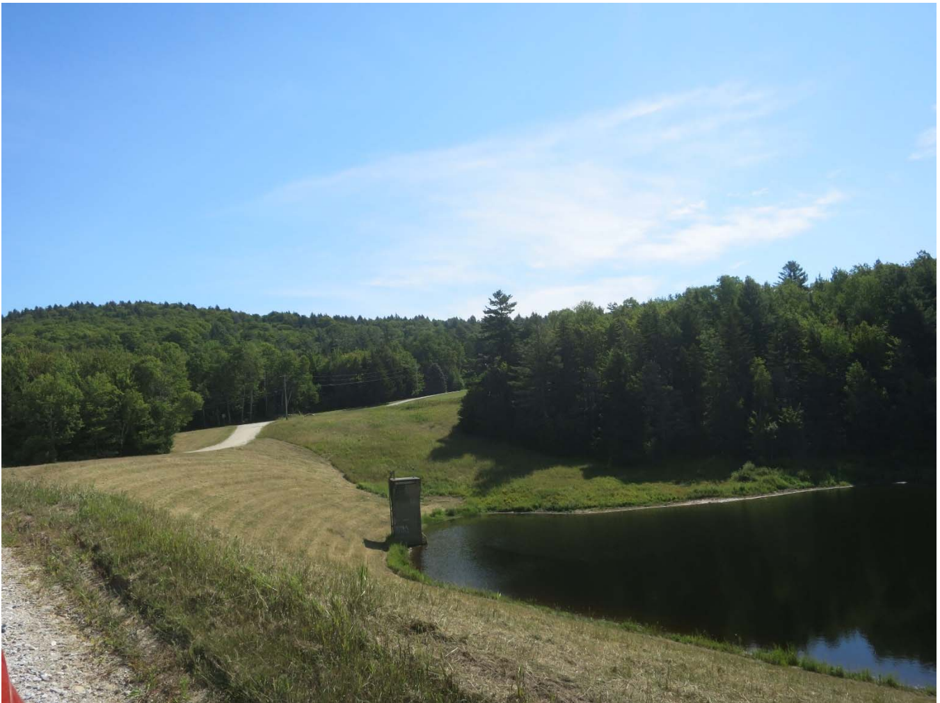
3. View east, showing the approach road, at center left, and the intake structure, August 2022.
