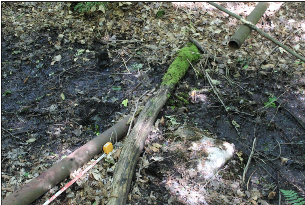
Photo 7. Dam 2, eastern pipe alignment crossing water collection ditch, in the east end of the APE. View to the south/southwest.
