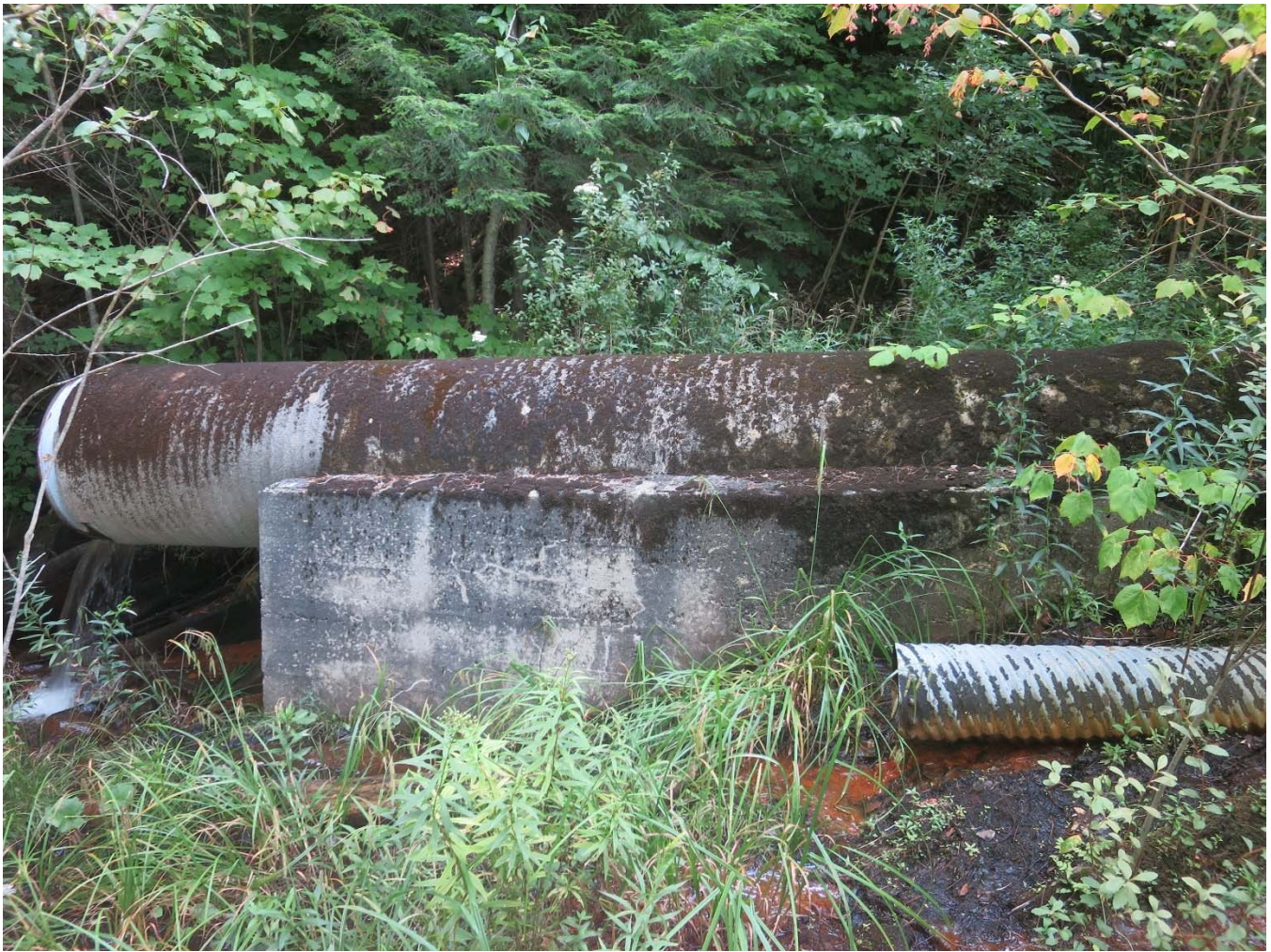
18. View south-southeast, showing concrete and corrugated metal outlet pipes, the former embedded in a concrete cradle, August 2022.
