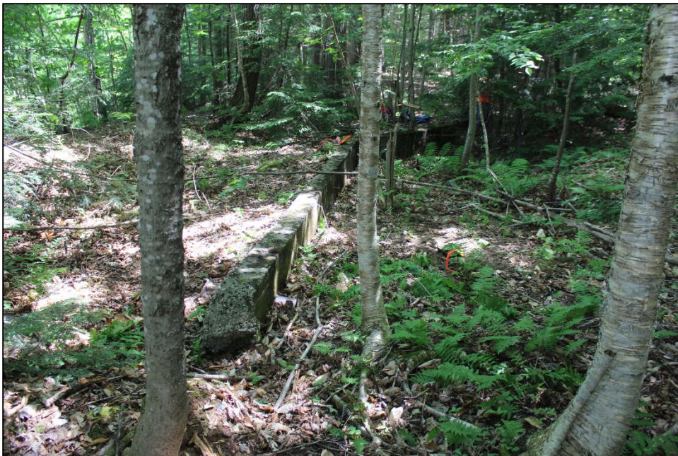
Photo 5. Dam 2, north end of ditch system with concrete wall forming the north side of this ditch, in the west end of the APE. View to the east.
