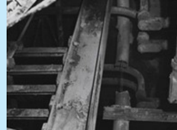
Browns Ferry 1 cable spreading room with melted aluminum cable conduit.
