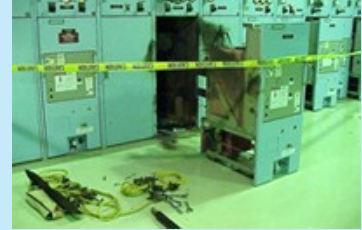
4-kV Switchgear at Browns Ferry 3
