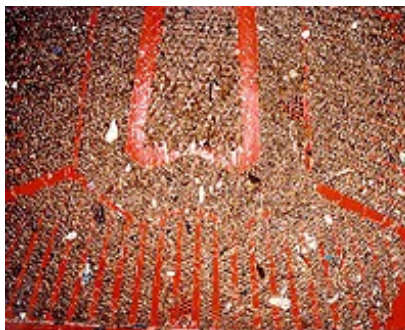
Condenser Tube Sheet
