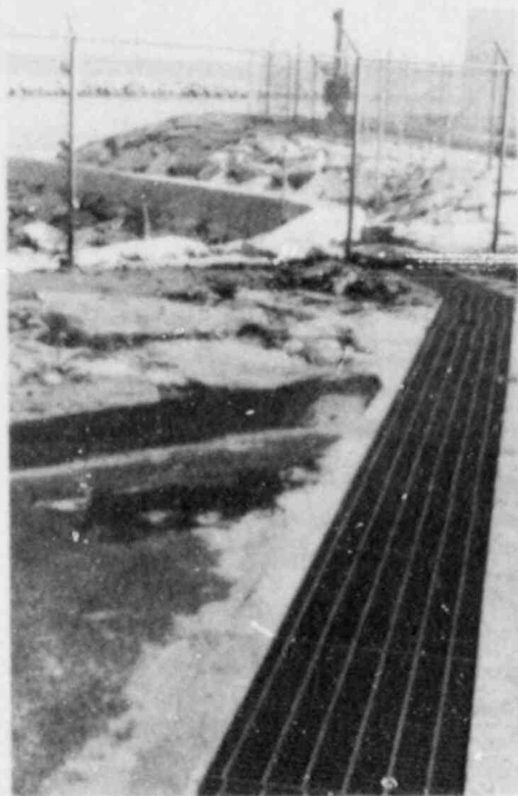
Plate 1. The 300 foot long Pilgrim Station, concrete screenwash sluiceway is molded from 18" corrugated metal pipe, and meanders over breakwater rip rap.
