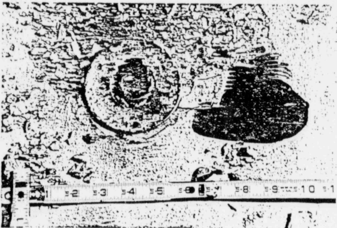
TYPICAL SHEAR FAILURE
