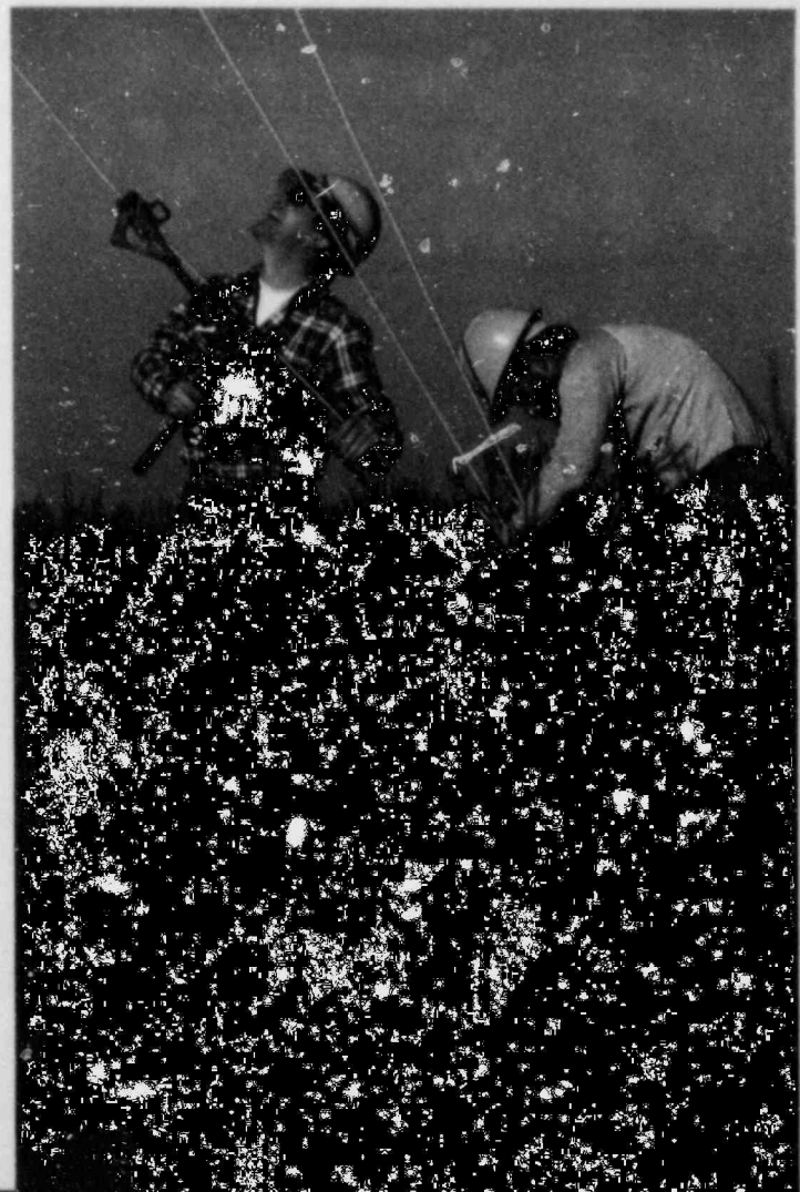
▼ Along a new transmission line, installed to further strengthen our transmission and distribution network, guy wires are carefully secured to support a large pole. Nearly 29,000 miles of lines now cover our System.
