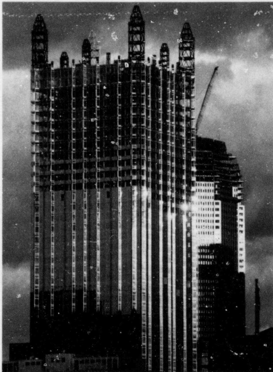
Pittsburgh currently is in the midst of Renaissance II—a multi-billion dollar project involving public and private construction work in the greater downtown area. PPG Place (foreground) the 40-story future home of PPG Industries, will dominate the city's new skyline, which will include six other skyscrapers by the mid-1980s.
