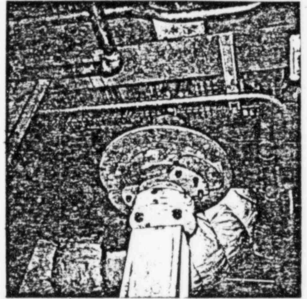
YOKE OPERATOR OF 1PSIBV402 ("E" HPSI Pump SUCTION L50)
