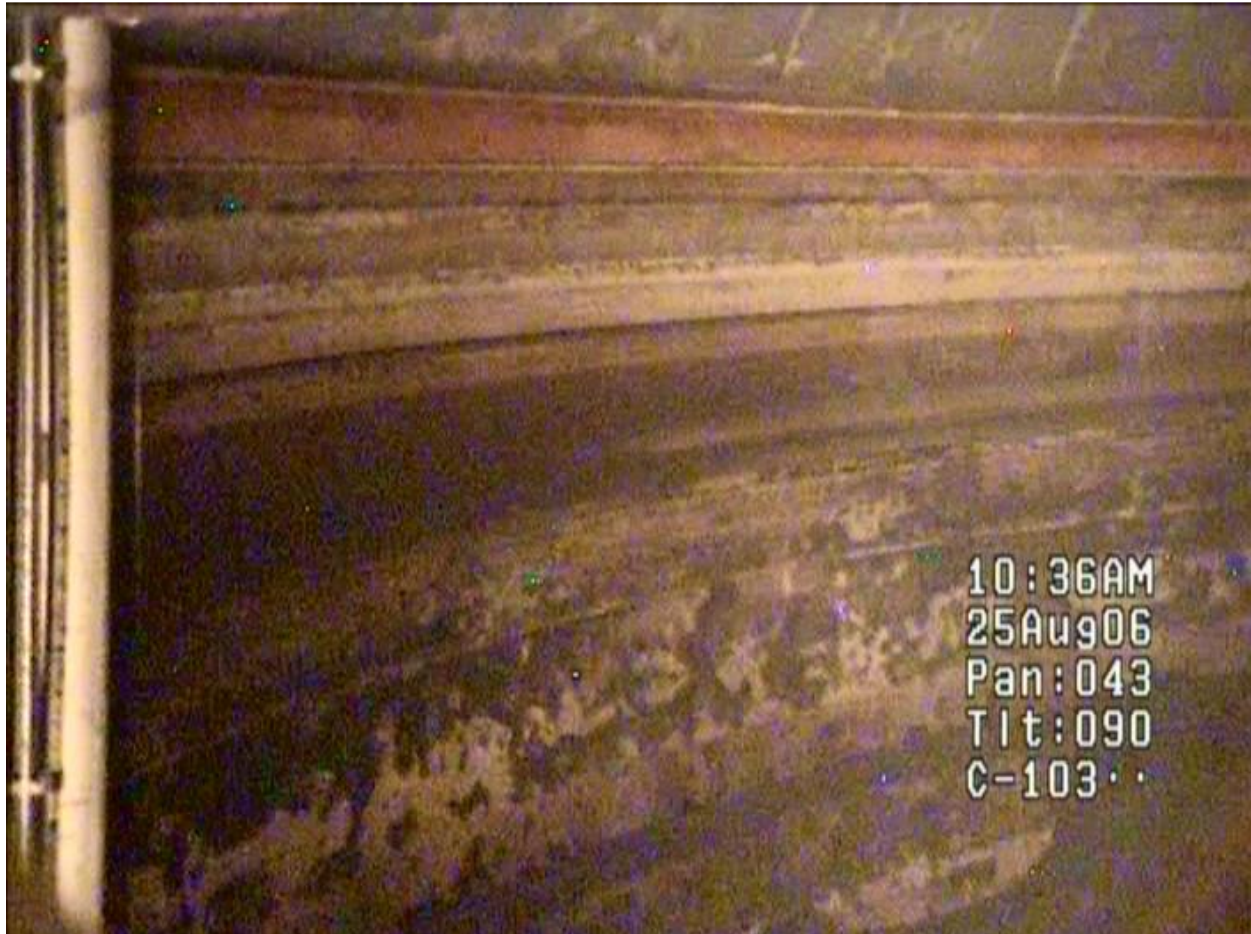
Figure 5-9. Tank 241-C-103 Waste on Walls and Stiffener Rings.
