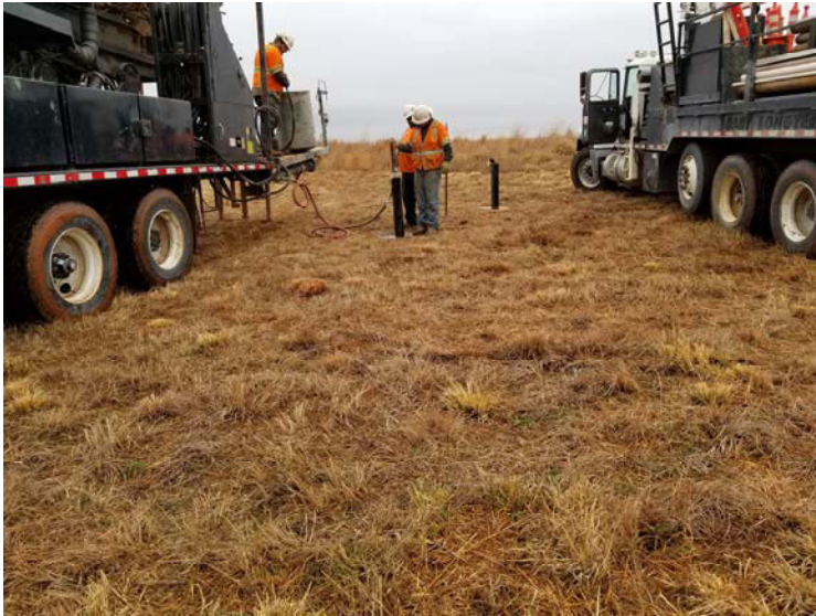
Photo 1: Tremie grouting monitor well
