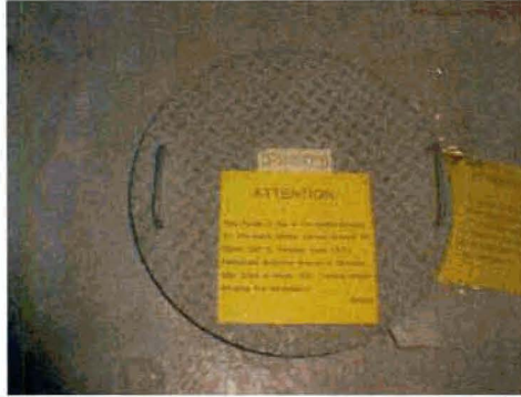
Photo1, P141S1028 Topside Room 1405 & Fire Area A-26
