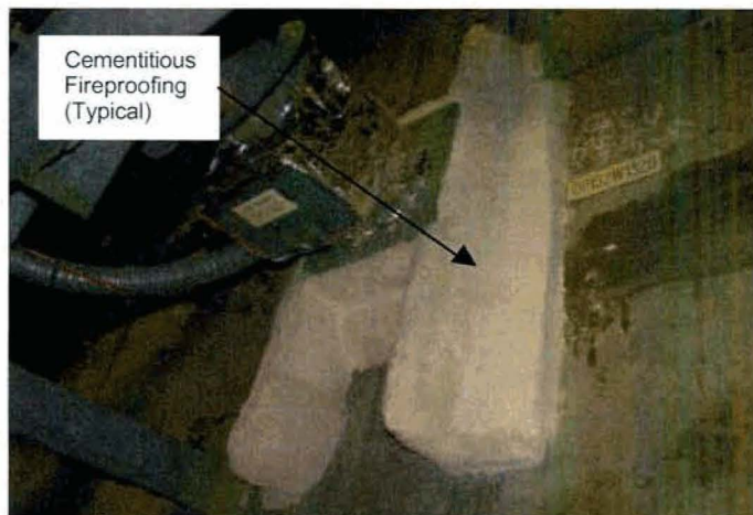
Photo 2 Fire Damper GKD0182 (from Auxiliary Building Side)
