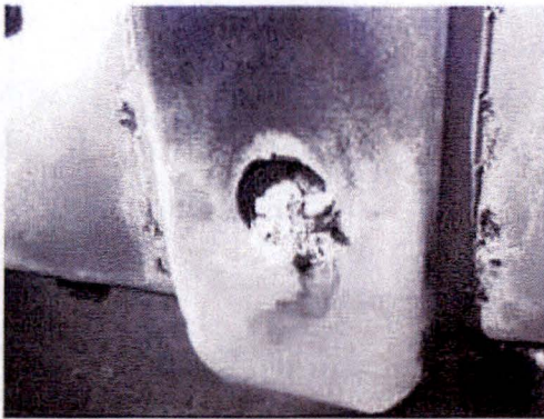
Figure 2.12.1-53 – Vent at stiffener
