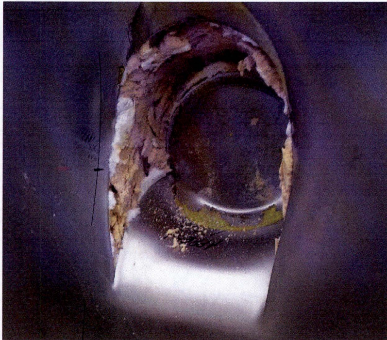
Figure 2-15 – Close-up of Puncture Damage for Test CP1
