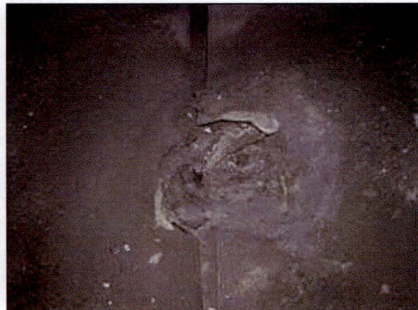
Close-up View of Puncture Bar Damage Area
