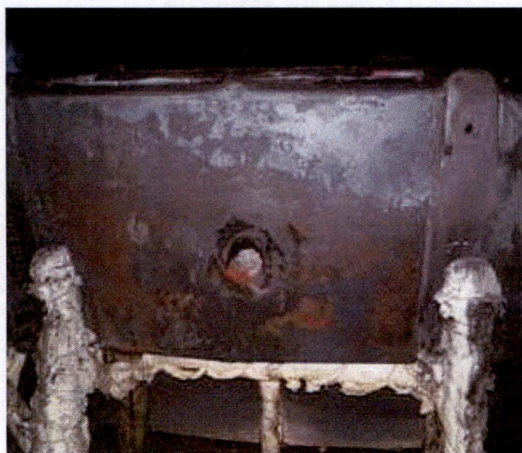
View of Puncture Bar Damage Area
