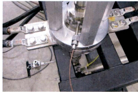
Figure 21: Lower Power Connection
