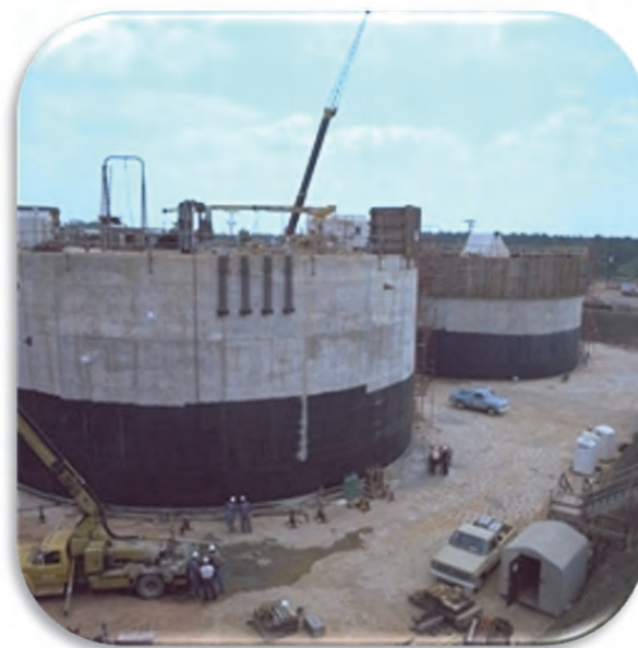
Tanks under construction. Note tank size relative to construction workers. Later, dirt is backfilled around the tanks to provide shielding
