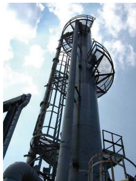
Figure 9-10 SRS Modified the M-1 Stripper System in 2007 to Remove Mercury
