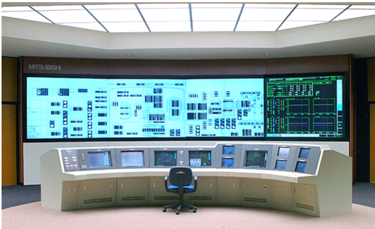
Figure B-2 The Facility Used in Development Phase
