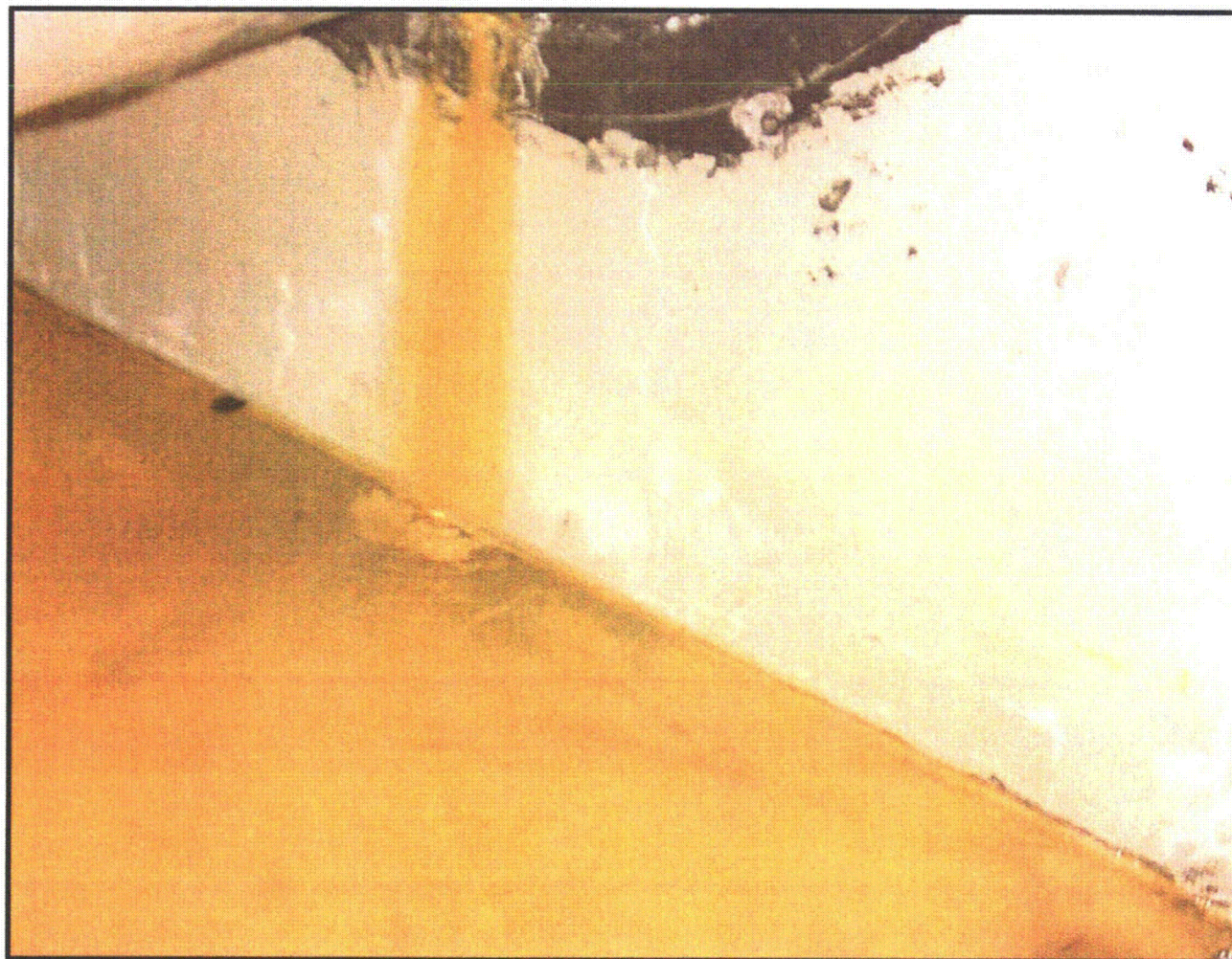
Photograph A-1. Fuel Transfer Tube Sleeve Leak in Unit 2 Reactor Building Photographed May 30, 2003.
