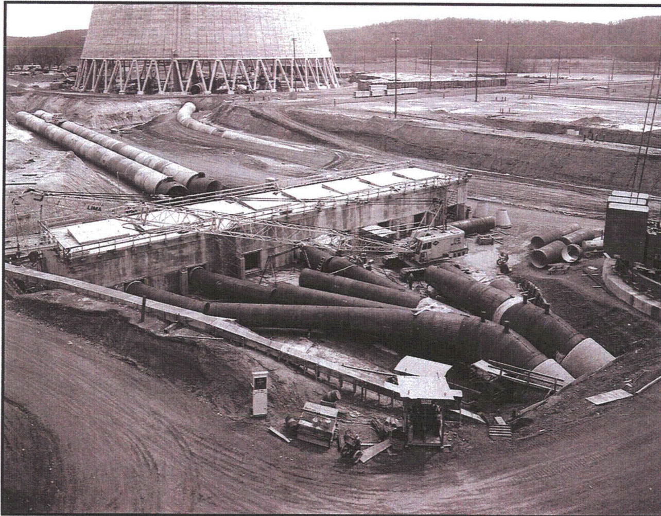
Photograph A-4. View east from Auxiliary Building toward Unit 1 Cooling Tower of the Condenser Cooling Water Intake and Discharge Pipe construction. Photographed June 1975
