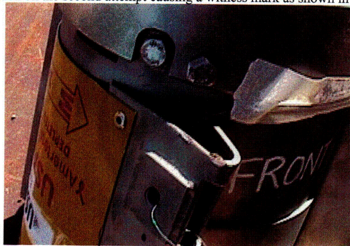
Figure 3: Penetration damage to cover bolt on TP84(A)
