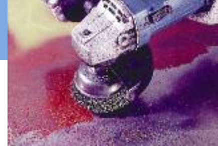
Removing paint from a steel surface with a crimped wire cup brush.
