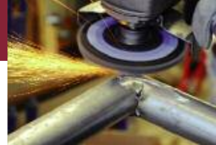
Weld blending on the corner of a security gate with a Tiger Paw XHD.
