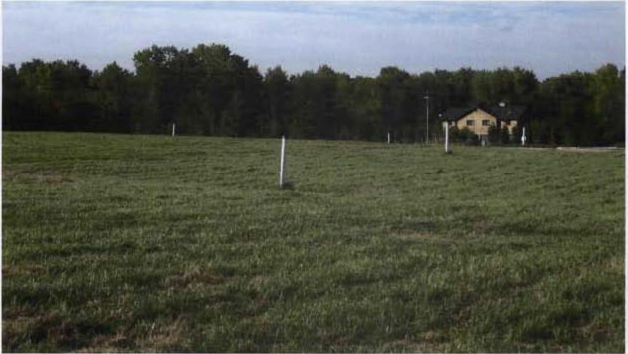
Landfill Cap, Facing North, slight depression with no signs of water ponding.
