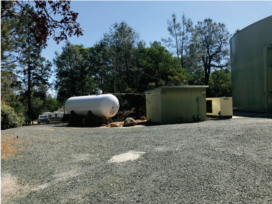
Existing pump station building, white pressure tank, generator and storage tank, northeast view
