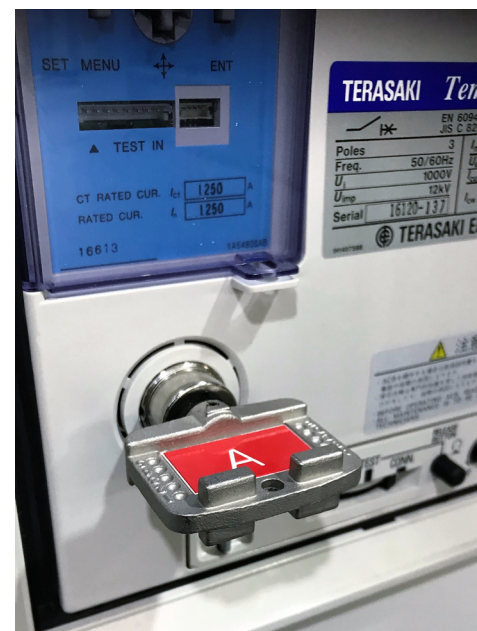
Figure 2 Trapped key lock with ACB cover fitted
