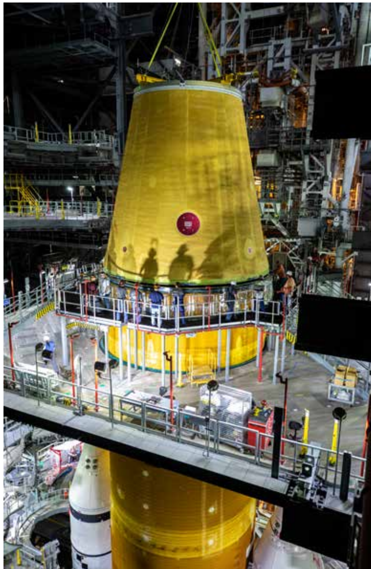
Jacobs crews bolt the launch vehicle stage adapter to the SLS core stage in the Vehicle Assembly Building.
