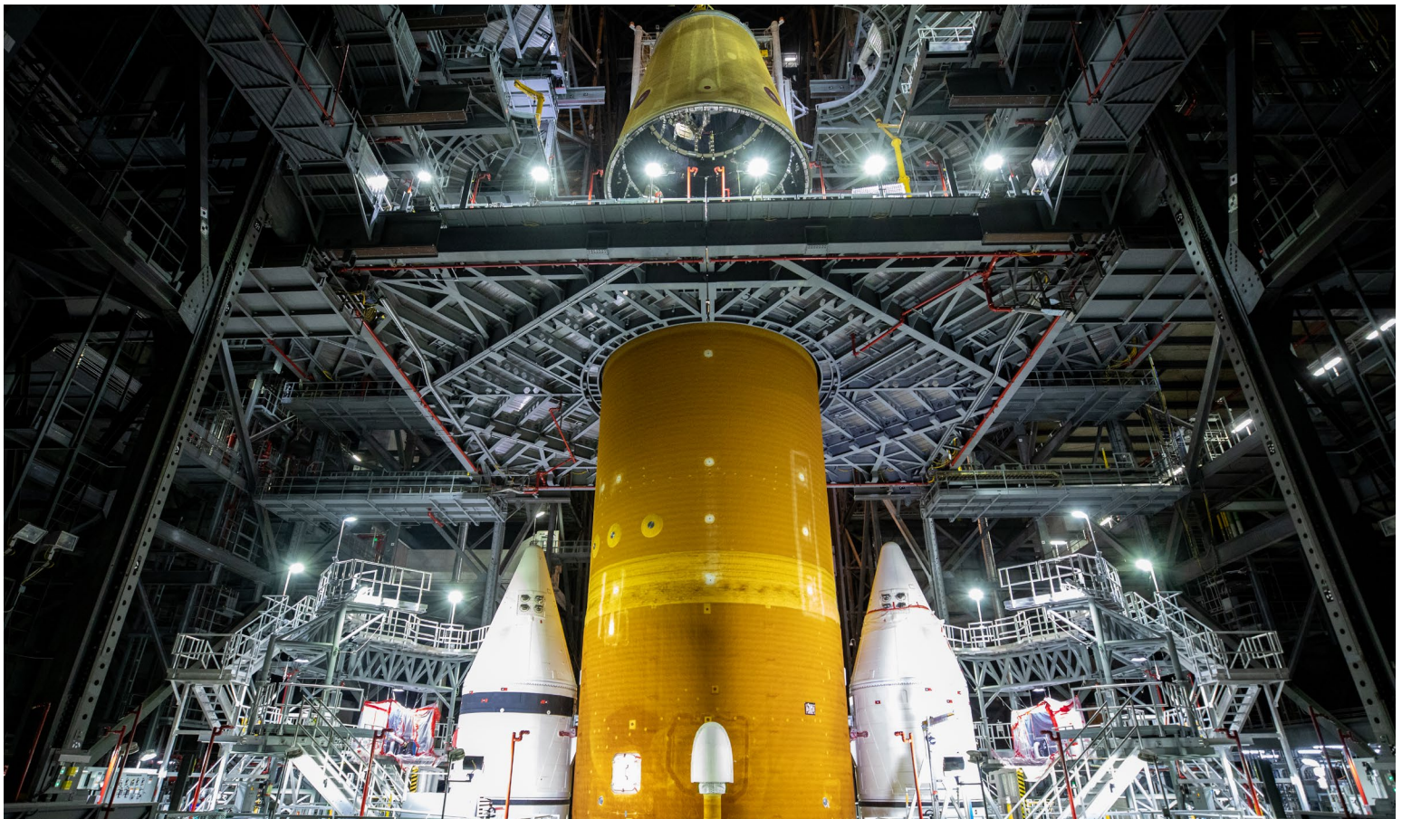
The SLS gets its signature orange color when its spray-on foam insulation darkens with exposure to sunlight. The core stage below the work platform was exposed to months of sunlight during Green Run testing at Stennis, while the launch vehicle stage adapter being lowered into place above the platform has been stored indoors since its completion.
