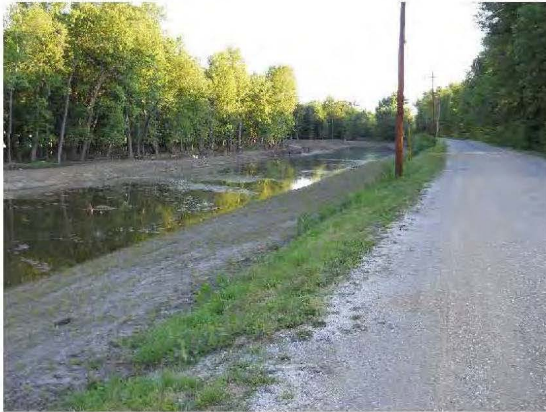
Discharge Channel excavation full after Illinois River water level crested at Minor Flood Stage
