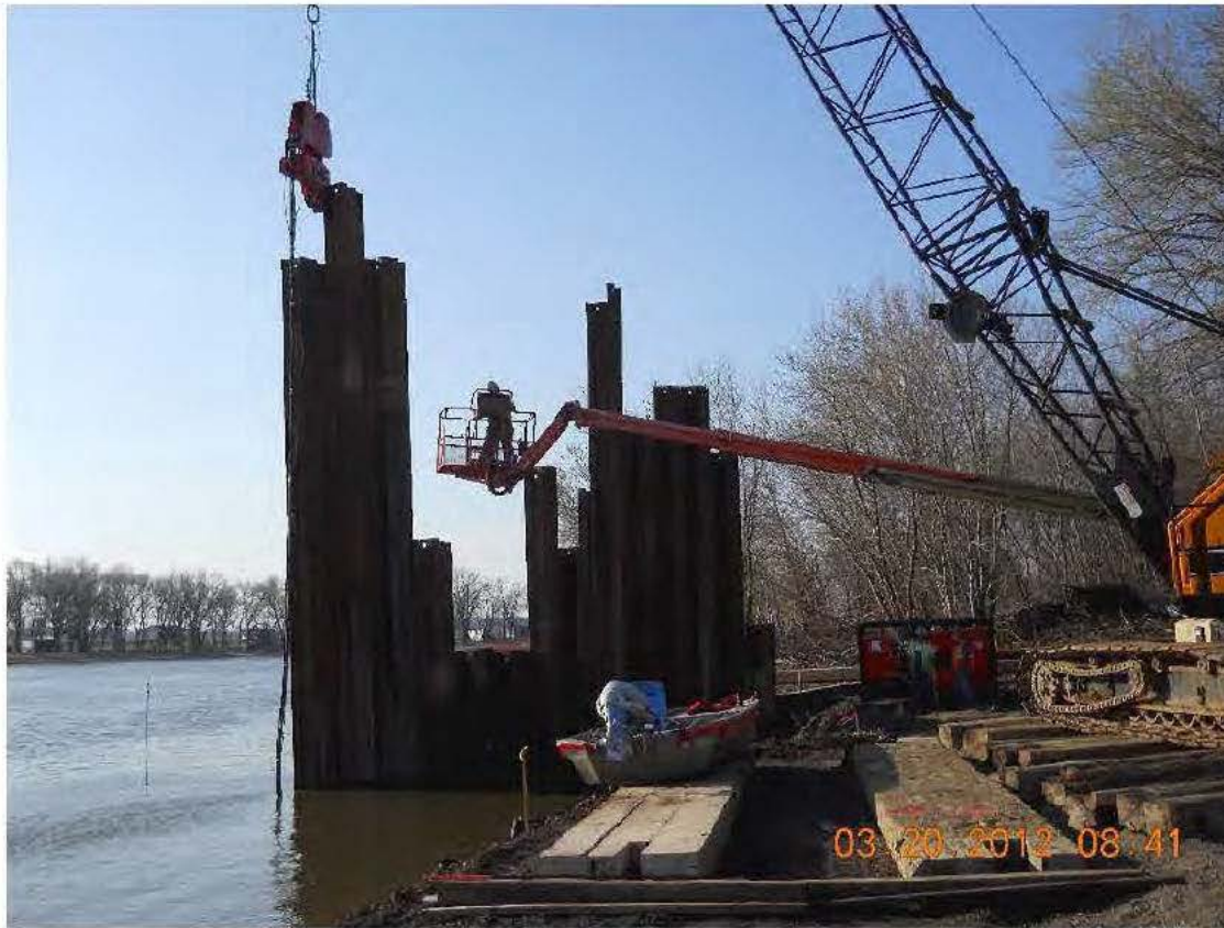
Sheet Pile installation for the cofferdam construction at the Pump Station Location
