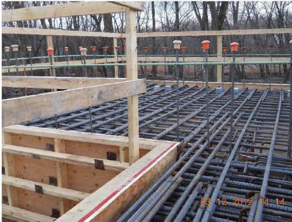
Control Building deck and support beam reinforcing steel in place and tied
