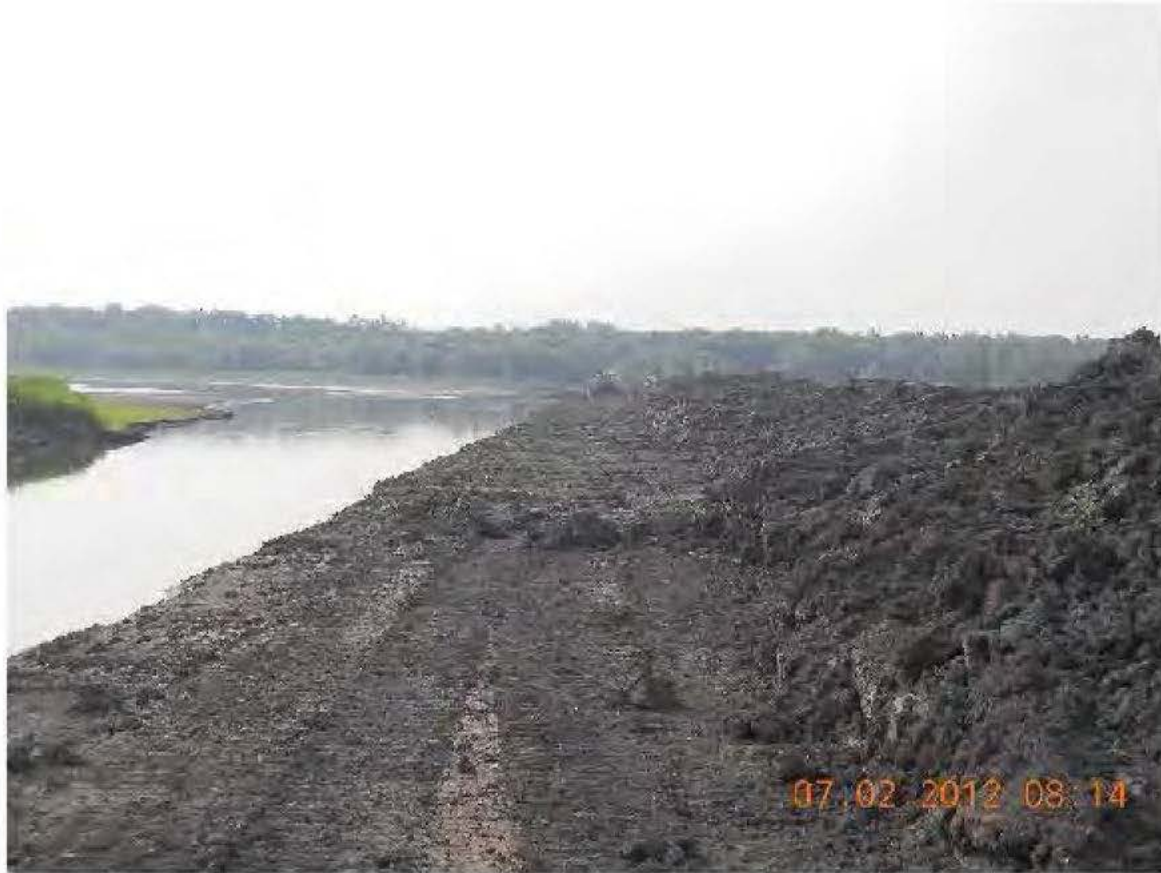
Overflow Spillway in the wet being aligned and drying for final grading
