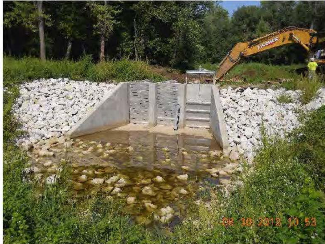
Outlet Structure Stop Logs and Gate installed. Excavation of Channel from Goose Lake in progress
