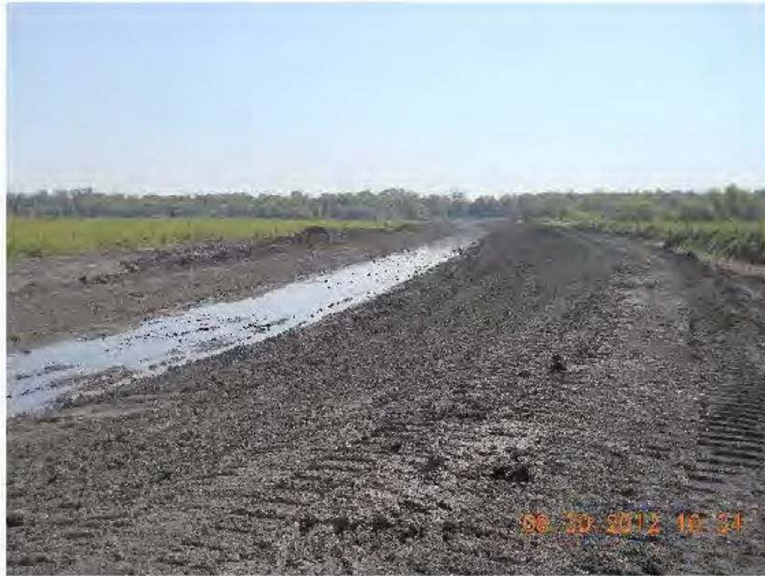
Discharge Channel Excavation and Construction at Station 40+00 looking East to Banner Dyke Road
