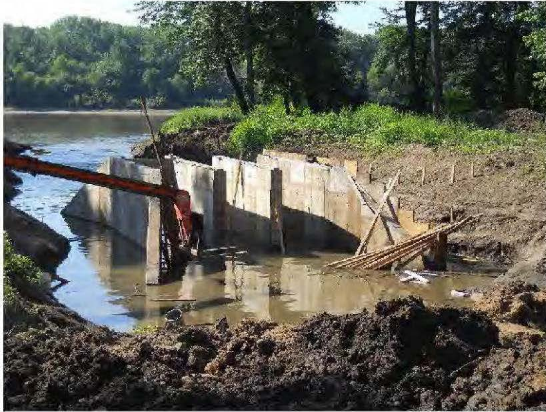
Forms being removed and area being cleaned around Outlet Structure after May flooding
