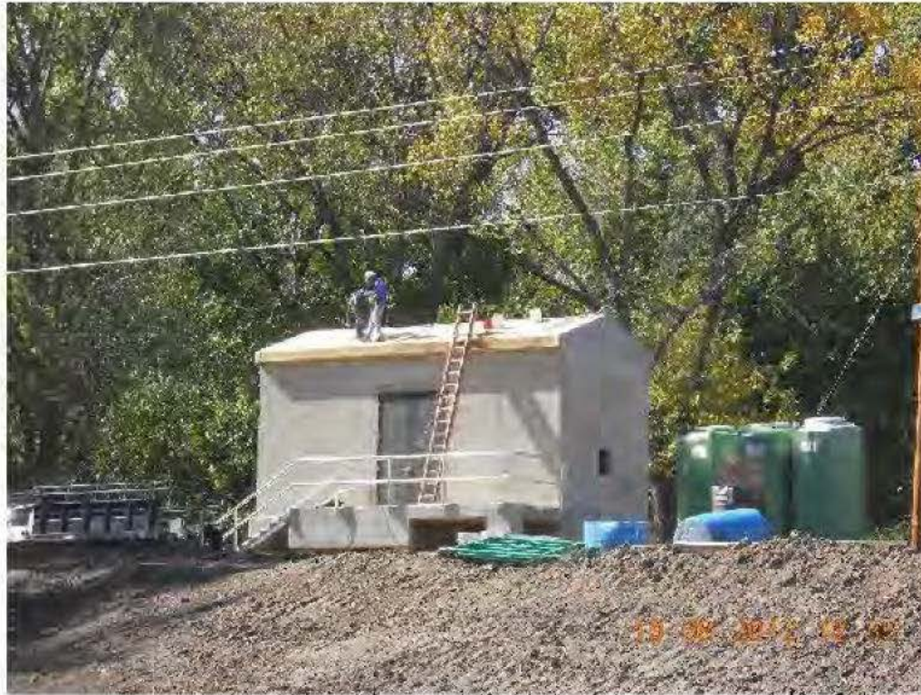
Control Building Roof Decking installation. Note doors and railing installation has been completed
