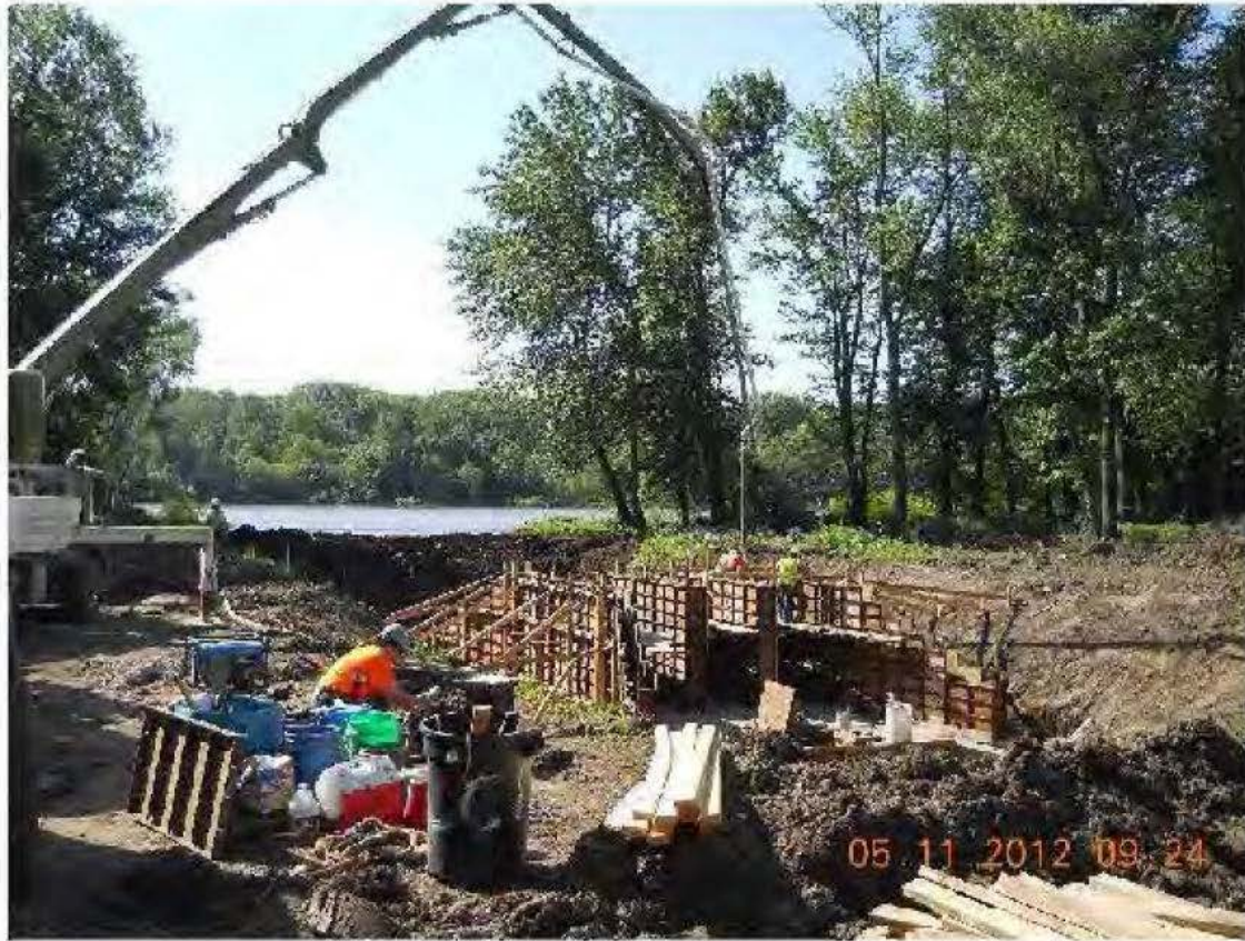
Wing Walls and Chamber Walls being poured at Outlet Structure from Goose Lake
