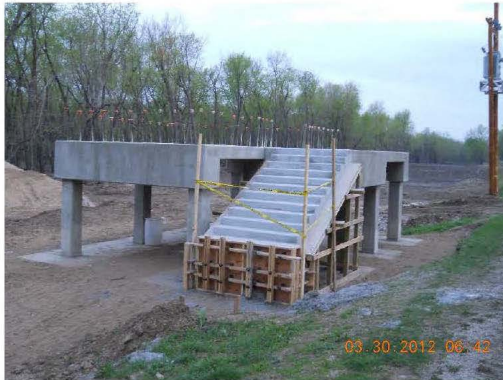
Control Building Steps poured and Side Forms Stripped. Support forms stay until concrete cures to required Strength
