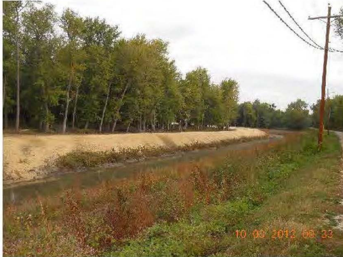
Discharge Channel Seeding approximately 50% complete. Photo taken next to Banner Dyke Road
