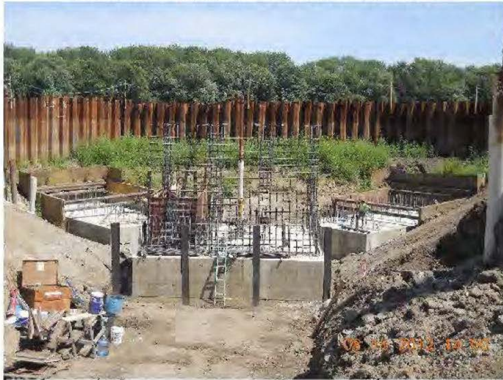
Pump Station Chamber Wall reinforcing steel placement begins. Foundation forms removed prior to backfill placement
