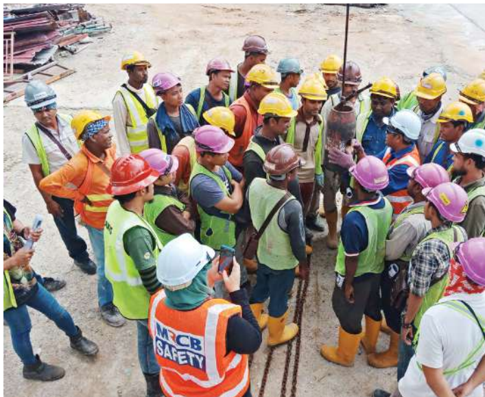
Daily safety "toolbox" sessions are conducted at construction sites to raise awareness of ongoing safety procedures
