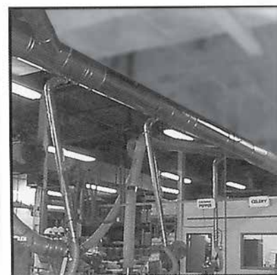
Straight duct from 4 to 22 inches diameter.
