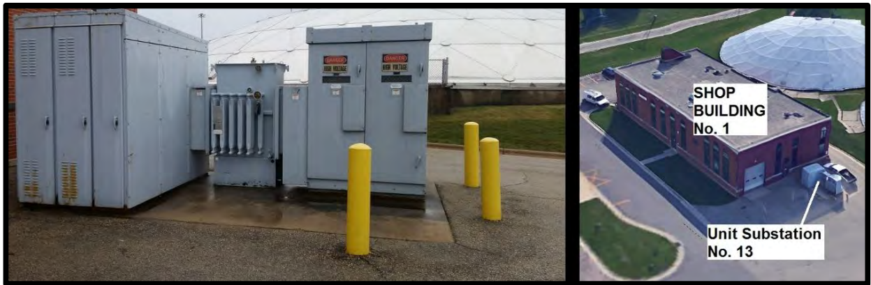
Figure 20—Unit Substation U13
