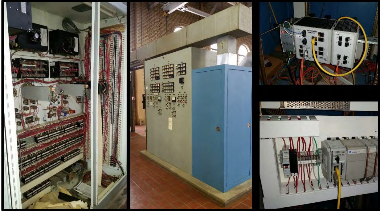
Figure 10–East Blowers Control Panel
