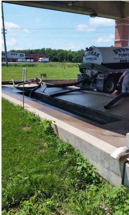
Figure 1 – Current septage receiving station
