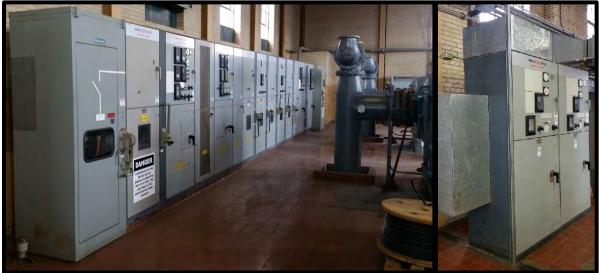
Figure 12–East Blower Building Medium-Voltage Switchgear (S141 & S142)
