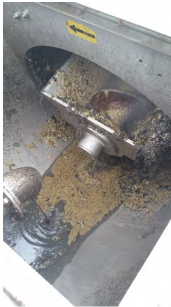
Figure 13 – Residual grease in inlet tank and trough
