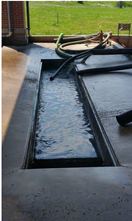
Figure 2 – Shallow slope in receiving trough
