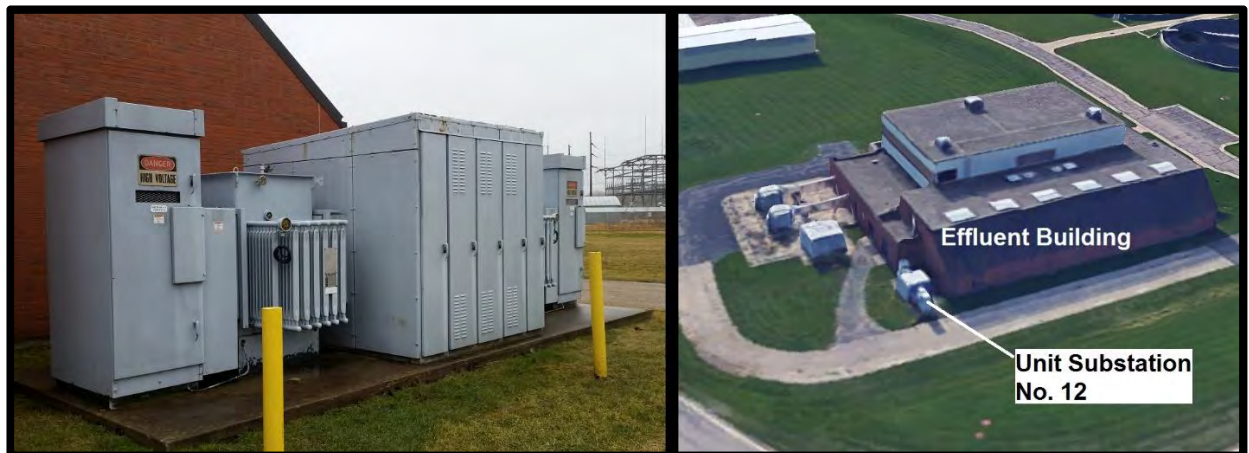
Figure 18—Unit Substation U12
