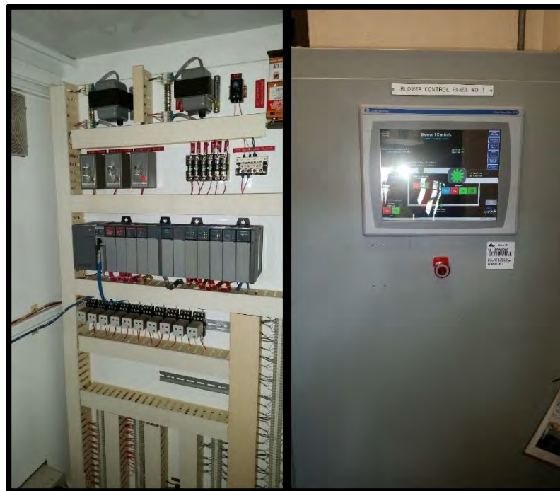
Figure 9—One of Three Upgraded West Blower Control Panels
