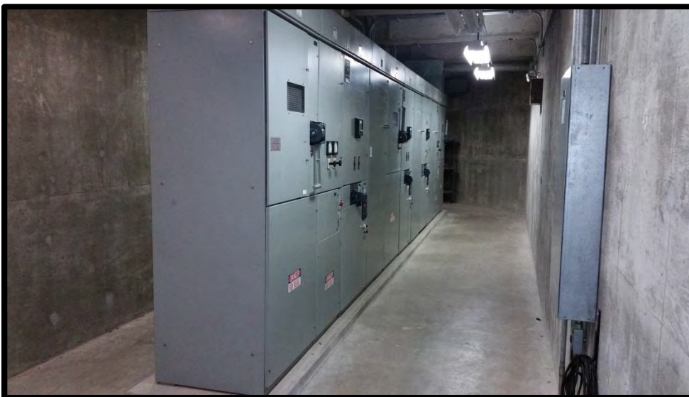
Figure 13–West Blower Building Medium-Voltage Switchgear (M51)
