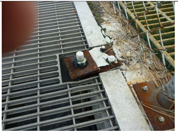
Photo 22 Outlet Weir operator plate.
