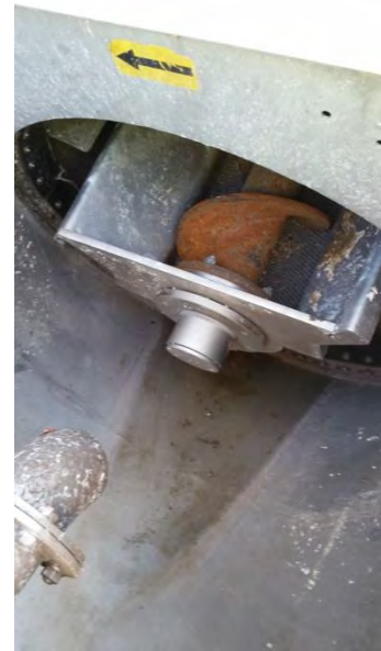
Figure 4 – Inlet tank and auger
