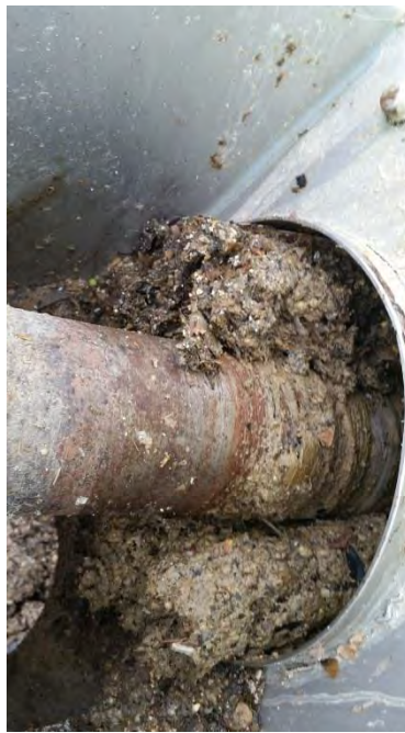
Figure 16 – Grease plug found in compaction zone
