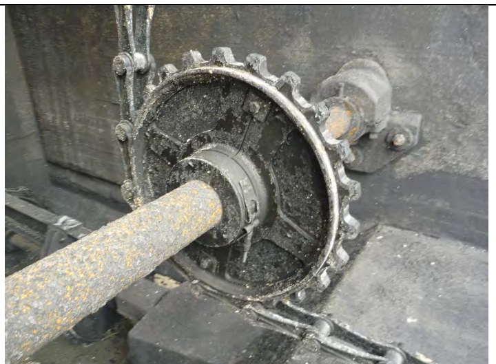
Photo 12 Primary Tank 1 drive shaft.
