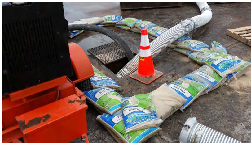
Figure 8 – Sandbags and pump were brought in to manage flooding
