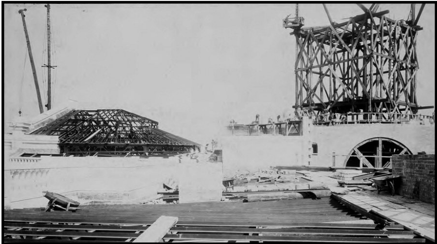
Two photos show the ironwork that forms the skylights above the chambers of the Minnesota Senate and Minnesota House of Representatives. One image (top) shows five men working above the Senate chamber on the west wing of the Capitol. Another photo (bottom) shows progress being made above the House chamber and dome. Both photos are from September 1, 1900.
