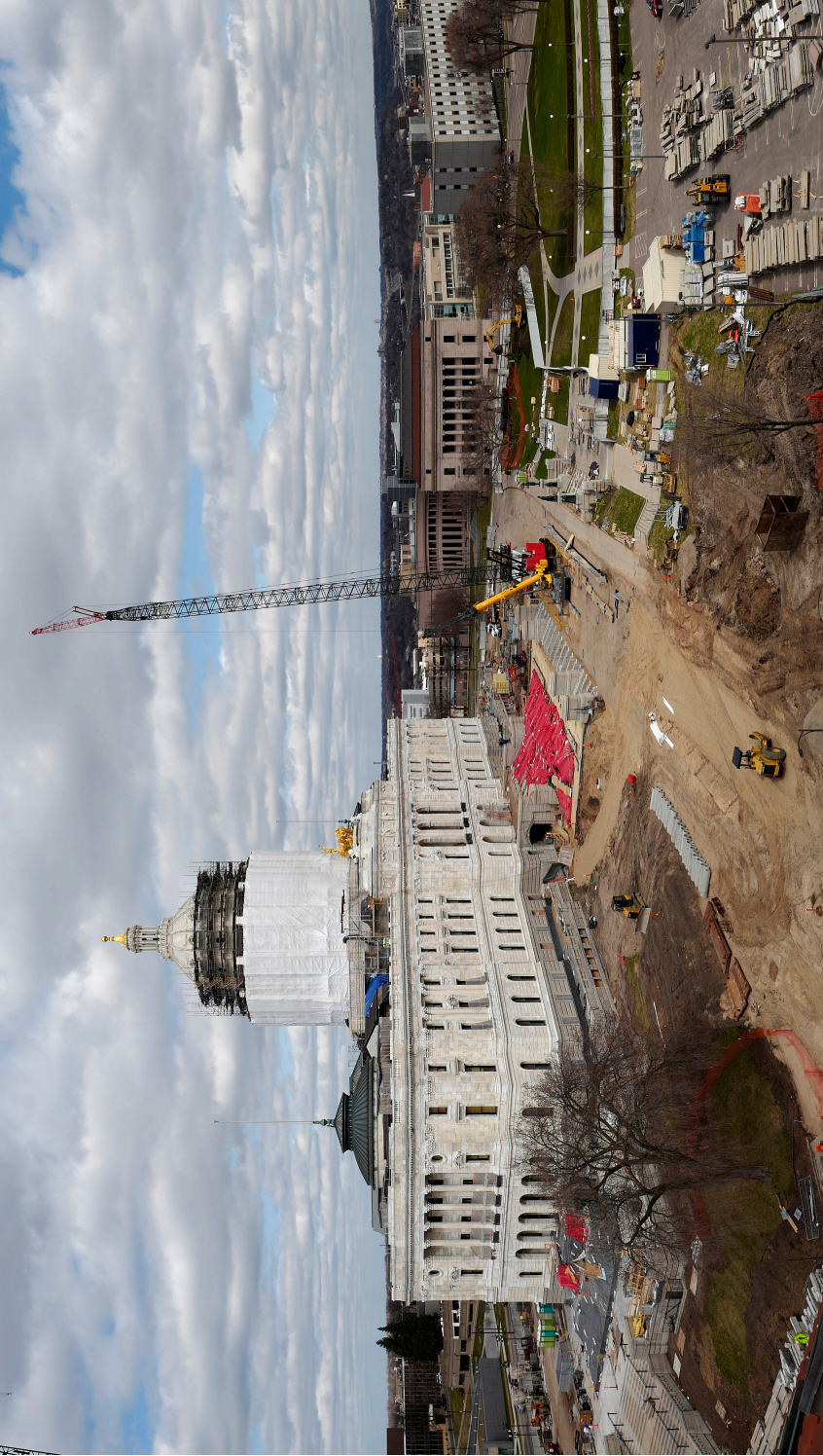
Aurora Avenue, the asphalt street, and parking were removed from the south side of the building to create a pedestrian promenade to link the Capitol to the Upper and Lower Mall.
