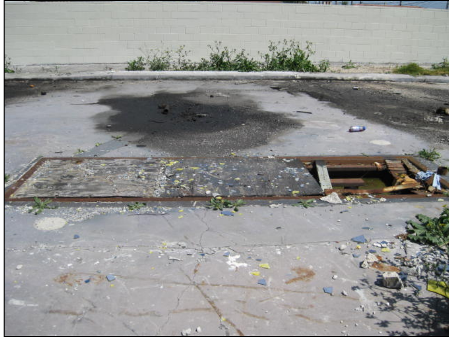
Photo 7: Photo facing east. Note the apparent oil/water separator located on the concrete pad.
