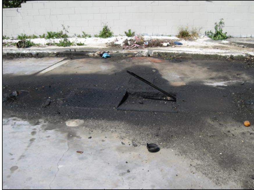
Photo 9: Photo facing east. Note the staining around the clarifier.
