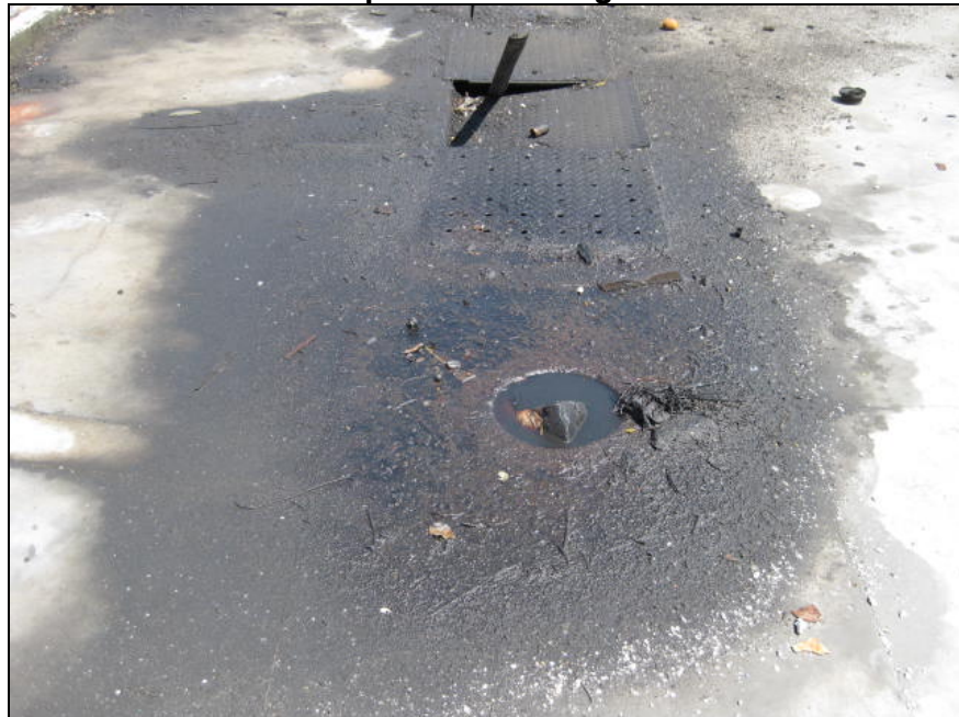
Photo 10: Close-up of the staining around the hoist.
