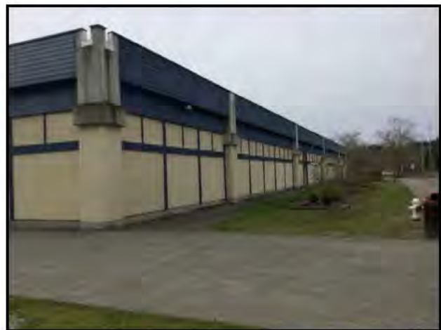
Figure 7-21. The north face of the main school building at 10601 NE 132 nd St., view southwest.
