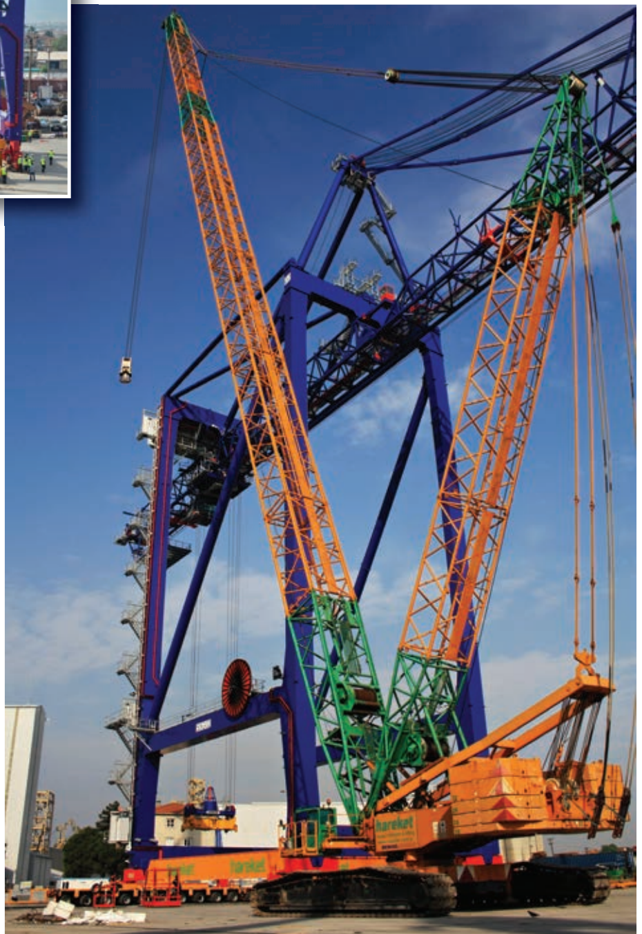
The cranes arrived at Derince port by vessel in sections and were assembled by the port's mechanical and electrical contractor Portunus
