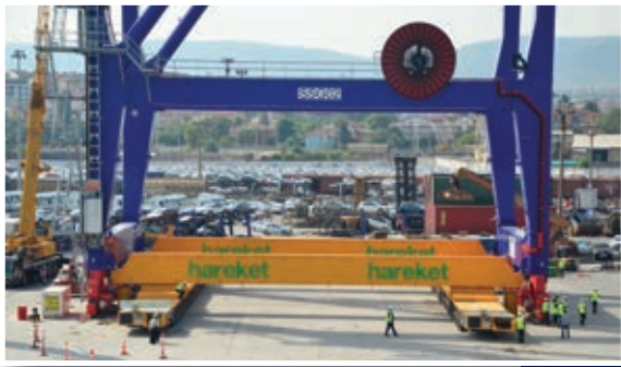
Two 28.5 m beams were put on the trailers to help transfer the weight of the crane
