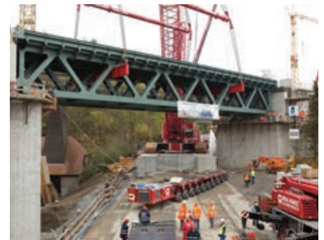
Positioning the 355 tonne load precisely on the abutments of the future railway bridge
