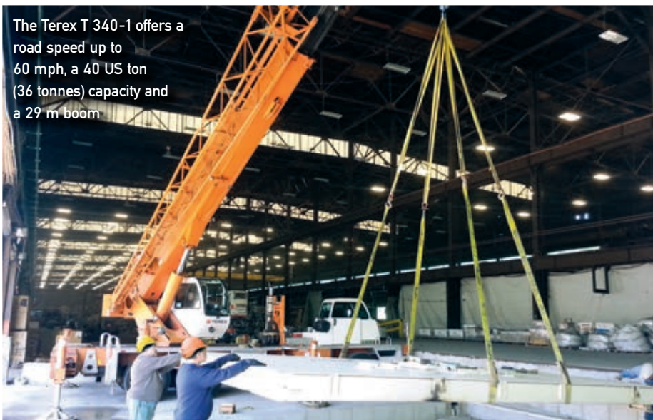
Zoomlion's new 110 tonne capacity QY110 truck crane on a five axle carrier
