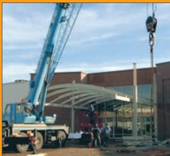
Members with the Hallenbau Huther GmbH company construct the overhang above the AAFES entrance Jan. 25 on Ramstein.
