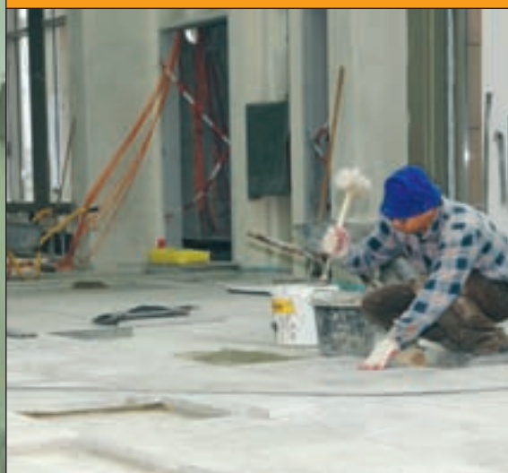
A worker for the German construction company, Bamberger, prepares the floor before laying the natural stone inside what will be the food court at the KMCC, Jan. 28.
