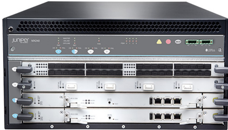
Figure 1.5 Juniper MX240 Router
