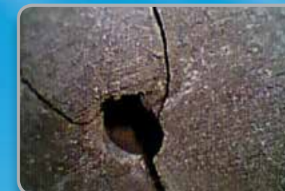
Using the Close-Focus tip, fine cracks are detected inside a combustion chamber.
