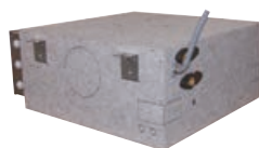
Metal parts insulated to avoid condensation
