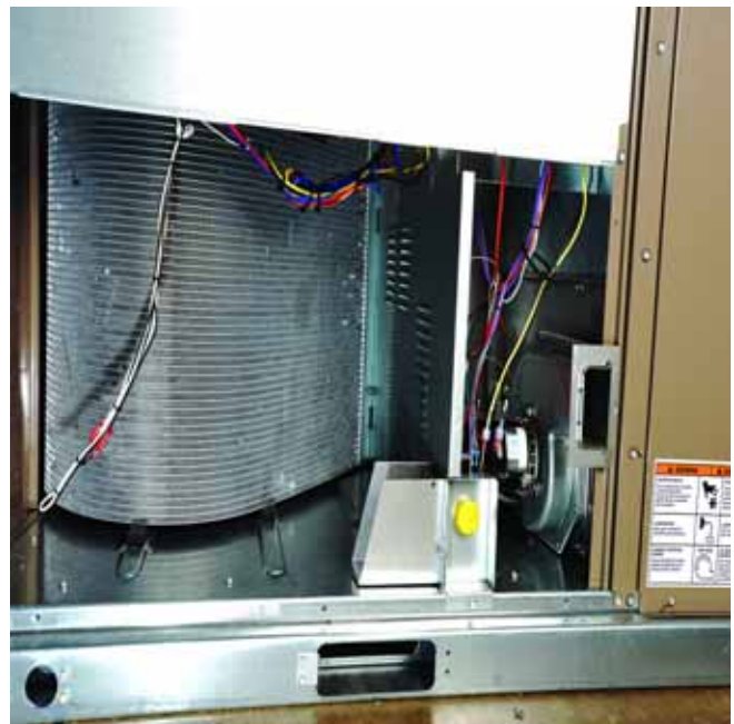
Figure 20: Flue Exhaust Hood Shipping Location
