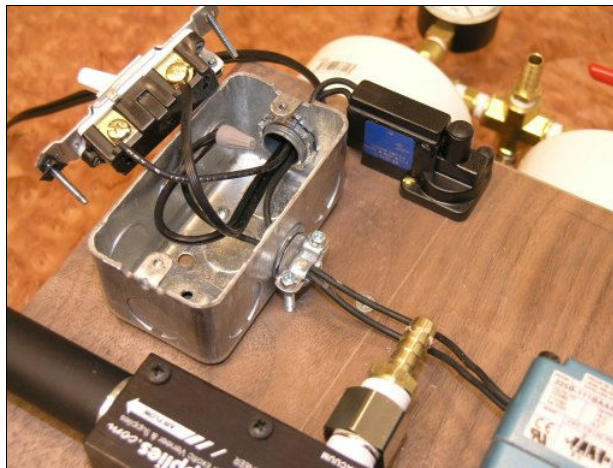
Completed Wiring of the Press
